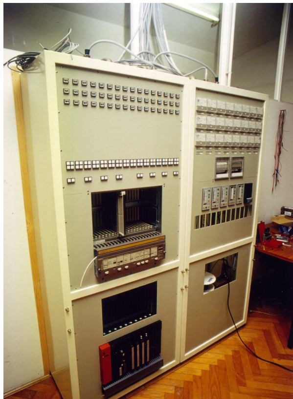
Fig 4. Classical control panel (under construction)
