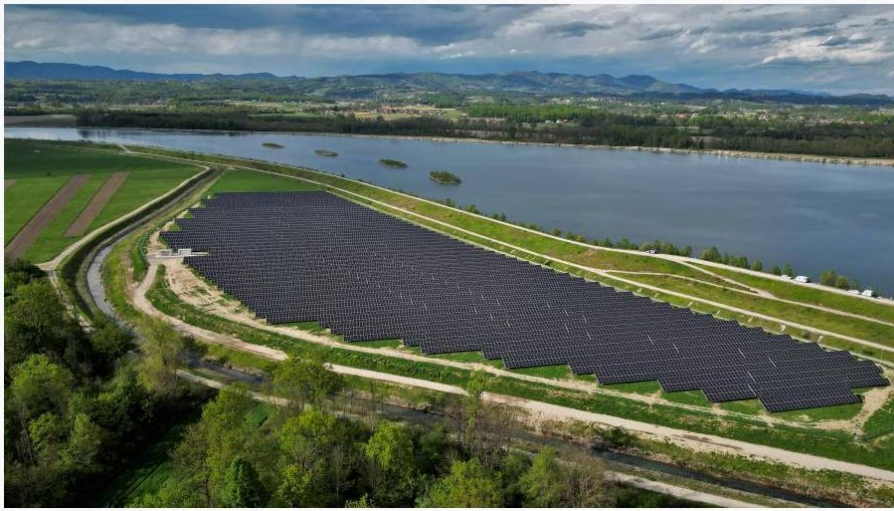
Figure 4.2: Case-study PV field [185].
